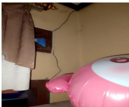
Figure 1. Hairline Crack Pattern on the Wall of a Resident's House in Neglasari Village
